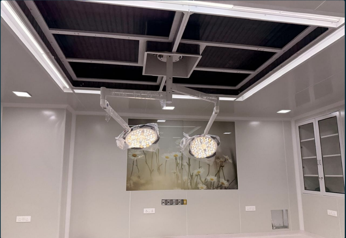
Twin Lumax 60 heads installed and commissioned in a live operating theatre
